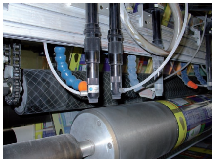
FIGURE 2: The advent of compact carbon dioxide lasers allows converters to use multiple lasers across a wide web. In this photo, each black tube contains the laser beam and focusing optics from a separate laser. (Photo courtesy of Alcan Packaging, Chicago, IL.)
